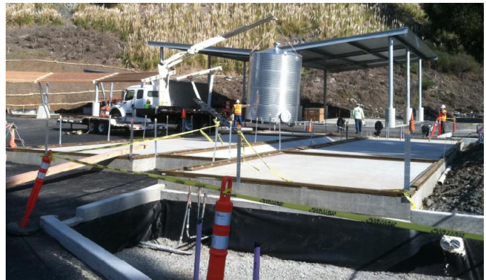
At El Cerrito's refurbished Recycling Center, a new cistern collects runoff to be used for irrigation and toilet flushing. In the foreground, a bioretention facility is being constructed for compliance with Provision C.3 in the Municipal Regional Permit.
